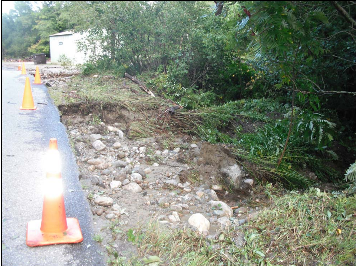
FIGURE 2. Peddler's Bridge Road Culvert Flood Damage & Town Shed in Ripton, VT ~ Aug 2011
